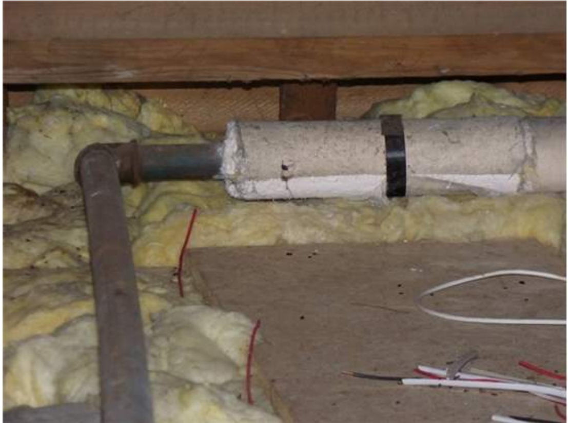
Lagging appears to be of an asbestos containing material (ACM)
